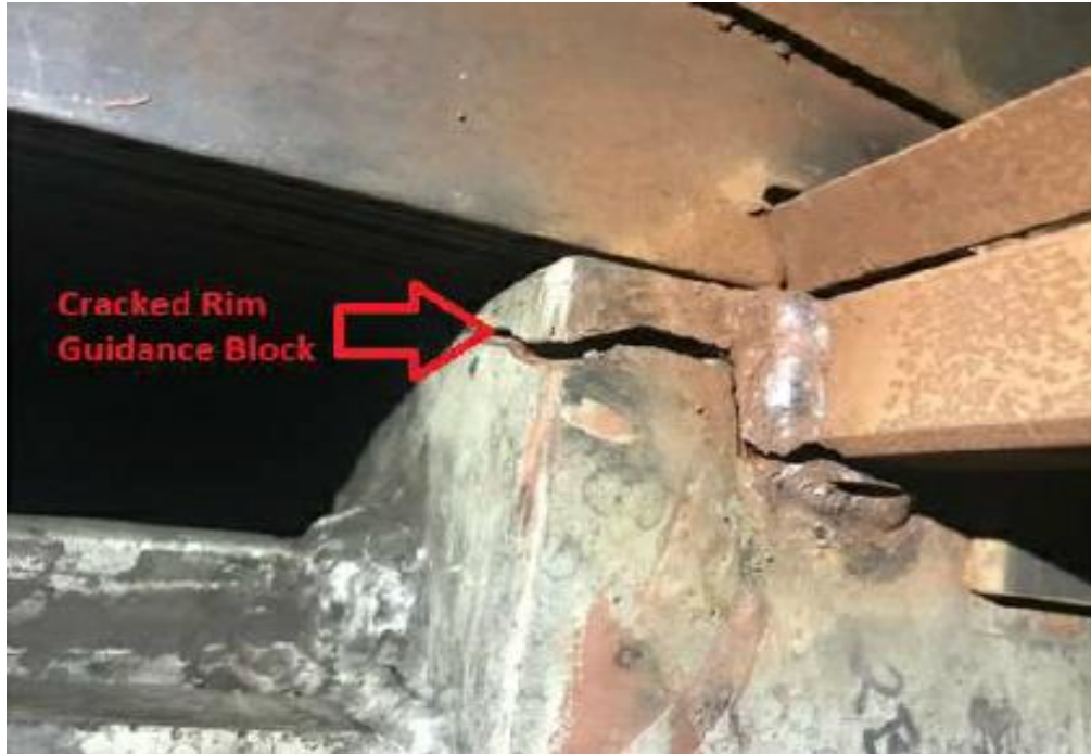
Figure 4: Rotor Rim Guidance Block #10 Crack
